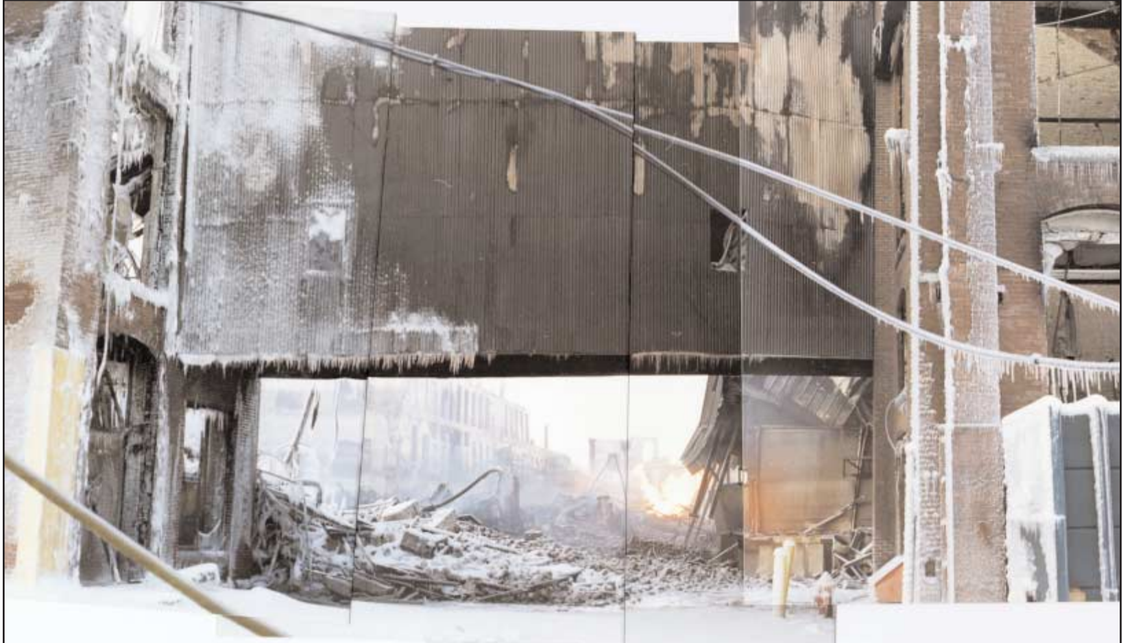
7. Composite of the overhead connecting bridge between the Monomac and Process buildings.
