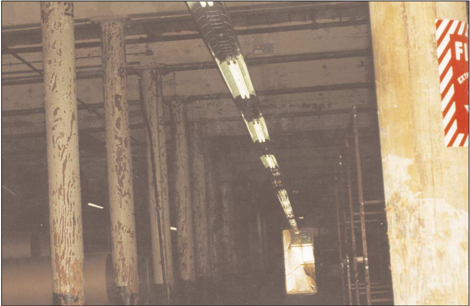
9. Typical mill building construction with heavy wood beams and thick wood floors.
