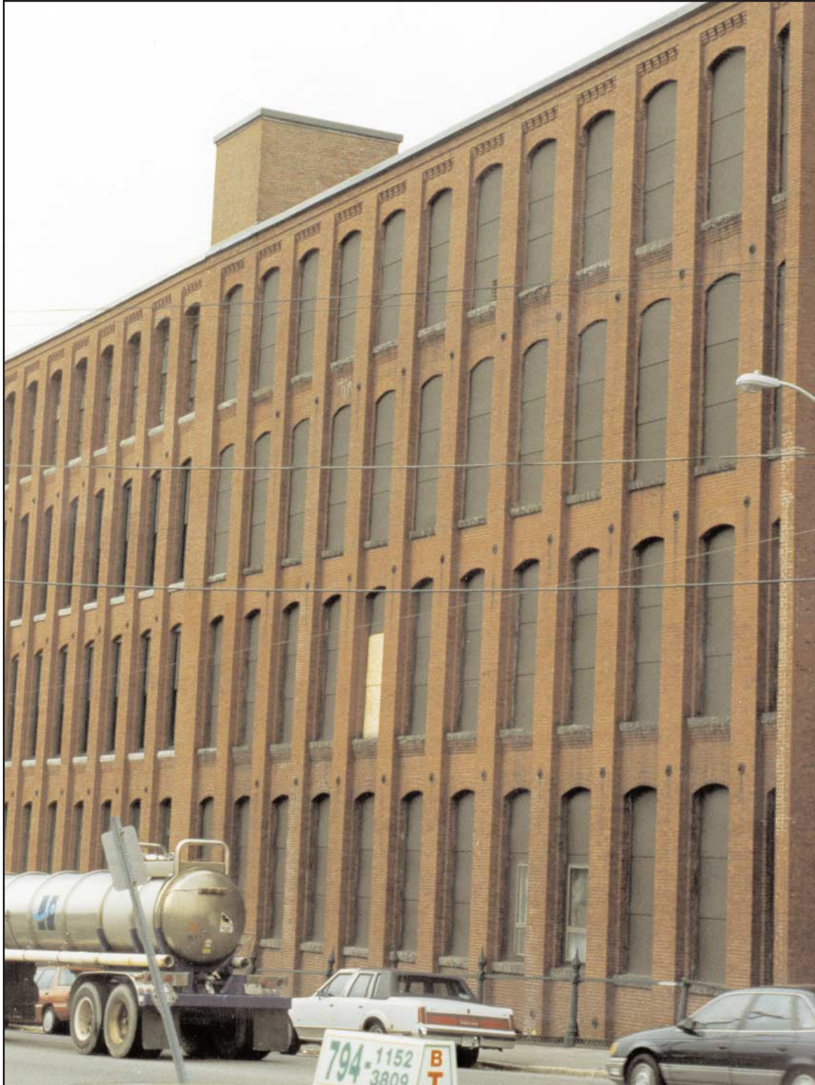
11. Windows once needed for natural light have been covered over, making visible fire location difficult. In addition, depending on the materials used, ventilation may be difficult.
